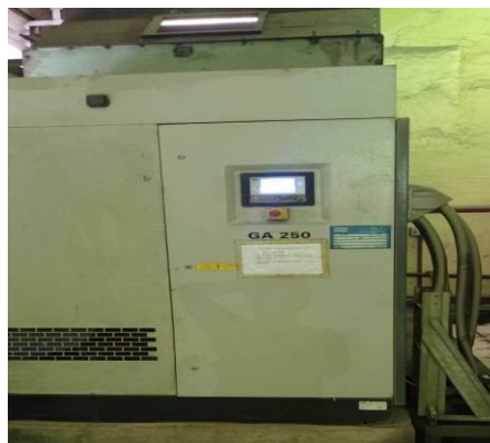
Gambar 3. Compressor Type GA 250 Atlas Copco unit Indarung IV
