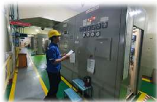
Gambar 3: Pengambilan Data Temperature Bearing Unit 2 PLTA Maninjau
