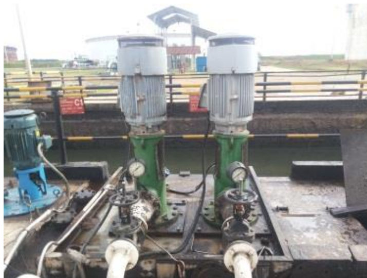
Gambar 1: Sump Pit Pump
